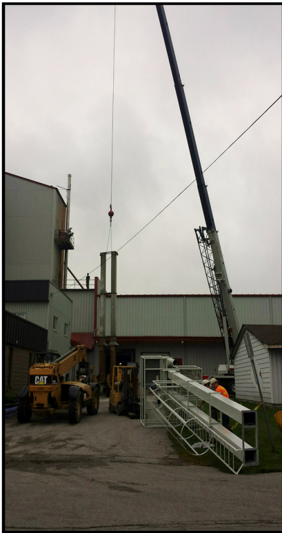
Jones Maintenance Staff install new elevator leg for the micronizers on September 2.
